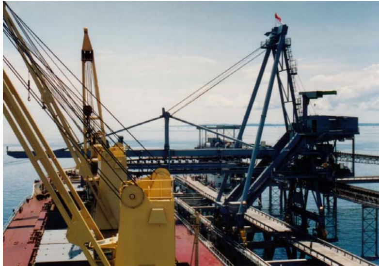
Figure 4 – 4000tph Shiploader Loading Capesize Ship
